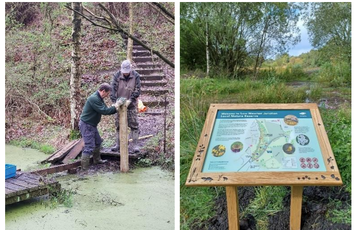
A new boardwalk and interpretation board have been installed at Low Newton Junction.
